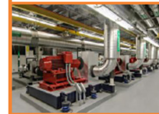
Central Utility Plant
