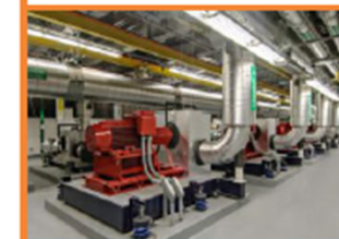
Central Utility Plant
